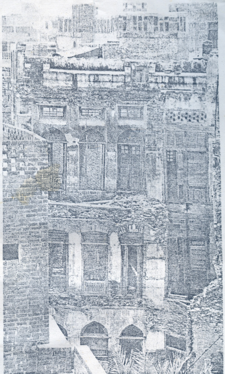
Majority of the dilapidated buildings are in the walled city posing a serious threat to the lives of those inhabiting them and those living in the neighbouring houses. Photos: Rahat Dar
